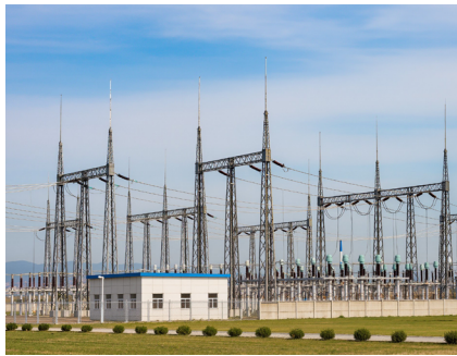
T&D & Renewable Substation
